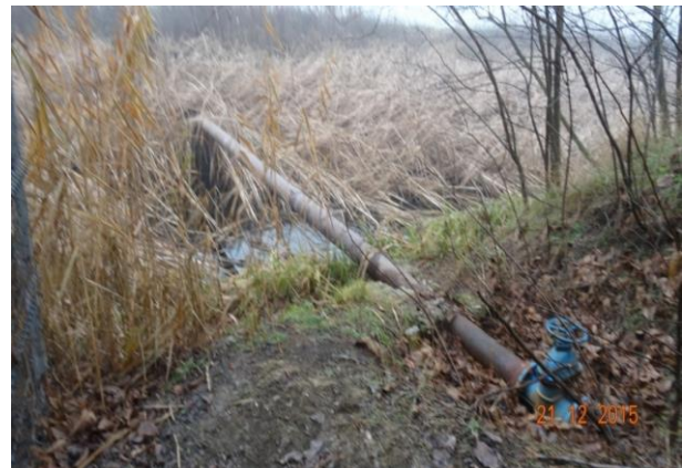
Figure 10 - Condition of the CA5 adduction channel with clogged sections and the presence of reed vegetation (Luca M., 2020)
