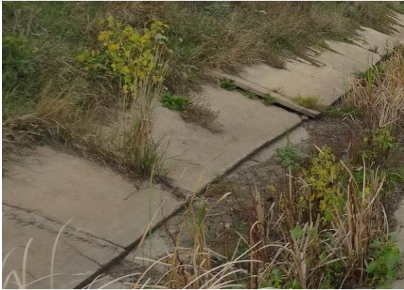
Figure 5 General structural conditions of the joints between the tiles of the CA3 channel (Luca M., 2020)
