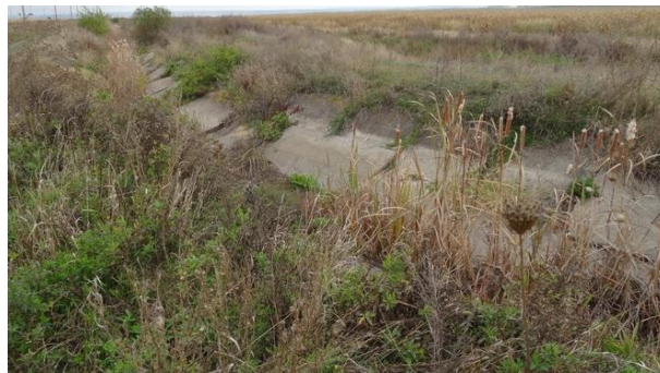
Figure 4 General structural condition of the CA3 channel between the SPP8 and SPP9 pumping stations (Luca M., 2020)
