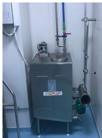
Figure 10 Brine production facility
