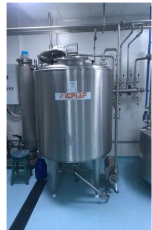
Figure 5b Buffer tank
