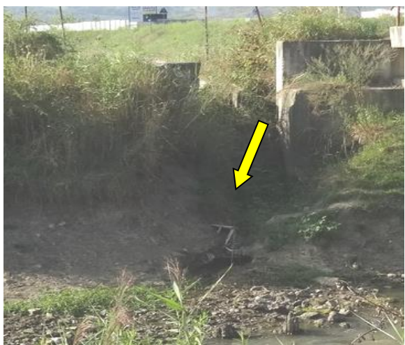
Figure 10 Intense phenomenon of erosion on the right bank of the Bahlui River bed at the outlet of perimeter channel 2 (Luca M., 2019)
