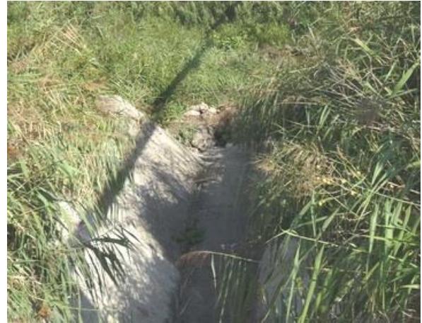
Figure 11 State of the evacuation sector (GV1) on perimeter channel 1 (Luca M., 2019)
