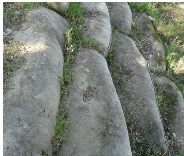
Figure 10 Degradation of geo-bags through cracks and tearing of material 2018 (photo author, 2020)
