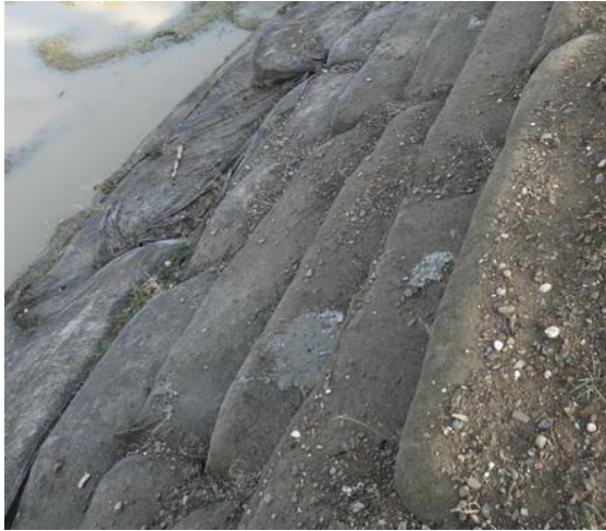
Figure 11 Degradation of geo-bags in contact with water in the flood of 2018 (photo author, 2018)
