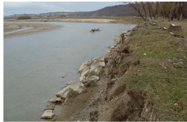
Figure 5 The total degradation of the defences on the left bank of the Moldova River, year 2012 (Luca M., 2012)
