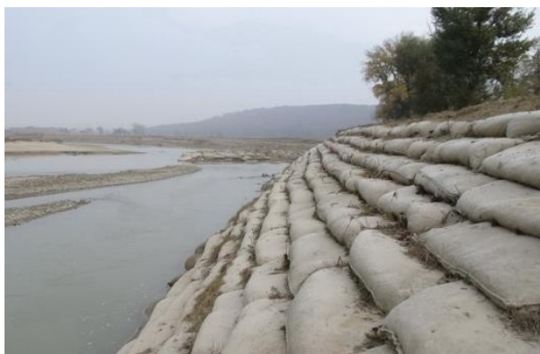
Figure 8 General view of the left bank defense after the 2016 flood (photo author, 2016)
