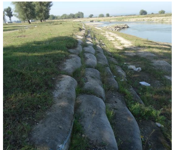
Figure 14 Coastal defence area with the presence of vegetation and alluvium deposits (photo author, 2019)
