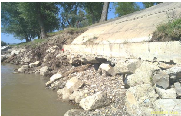
Figure 4 The structural state of the shore defence made of concrete slabs in 2008 (Luca M., 2012)
