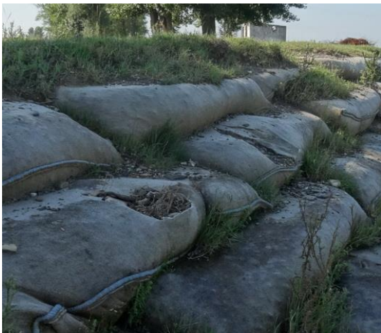
Figure 12 Degradation of the geo-bags located at the top of the coastal defence by anthropogenic actions (photo author, 2022)
