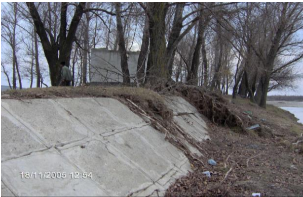
Figure 3 The structural state of the left bank defence on the Moldova River in 2005 (Luca M., 2006)
