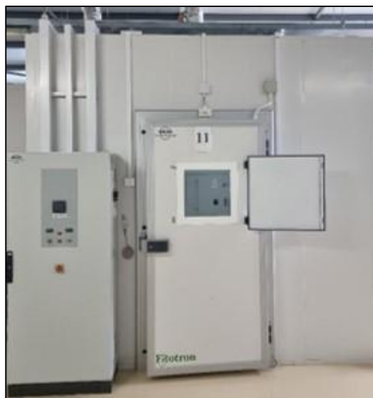
Figure 1 Walk-in Plant Growth Room
