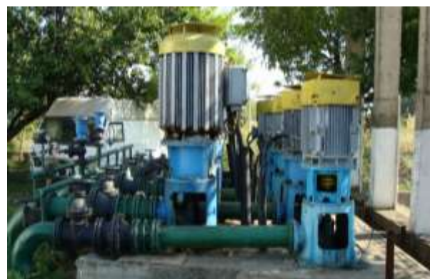
Figure 5 Hydromechanical equipment at SPP1b Soloneț South for bivalent watering (Luca 2012)
