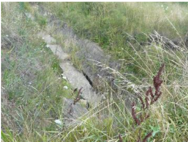
Figure 3 Tail-race channel made out of concrete is degraded
